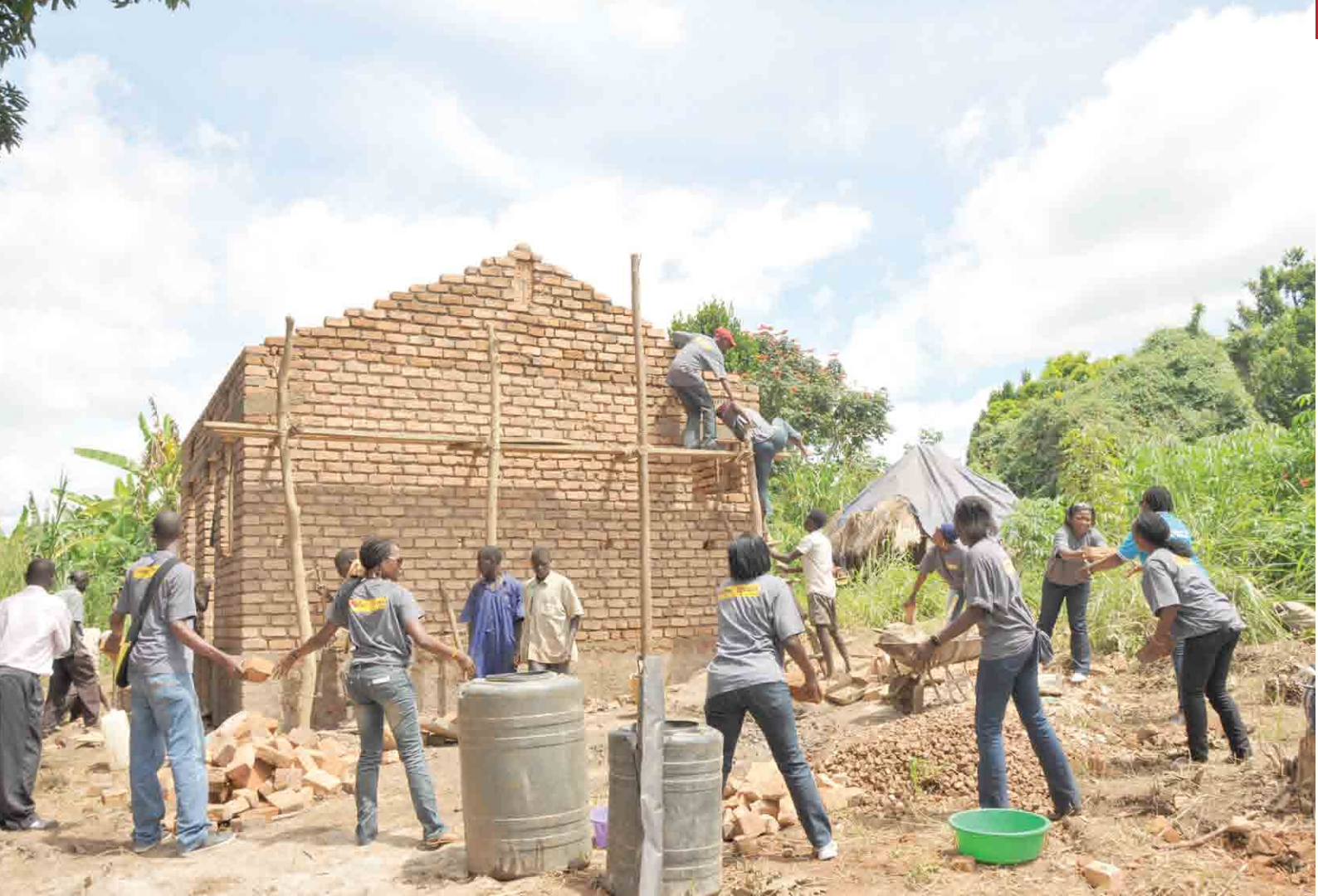
Vision Group staff construct a house for Nyakato, an HIV positive widow
